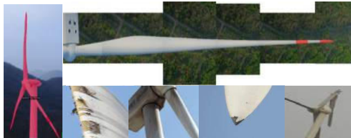
Wind inspection AI automatically recognizes the orientation of the wind turbine, and multiple captured images can be automatically spliced into complete wind turbine blades. The platform AI intelligently analyzes various types of defects in the wind turbine
