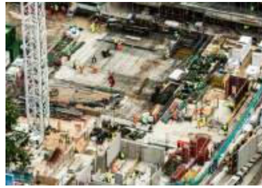
Identification and warning of vehicle intrusion around the site
