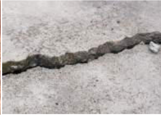
Ground cracking identification
