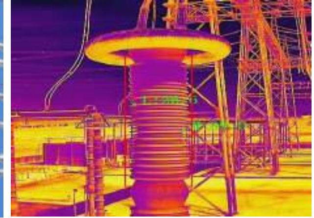
Intelligent temperature measurement at key positions of substation power equipment
